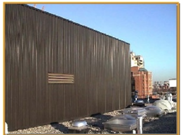
Solar Air Heating System on the Roof of Houghton Place Apts. in Cambridge, MA
