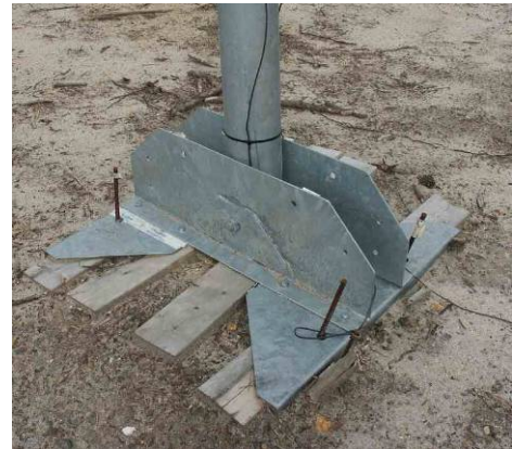
A met tower base-plate sits directly on the ground.
