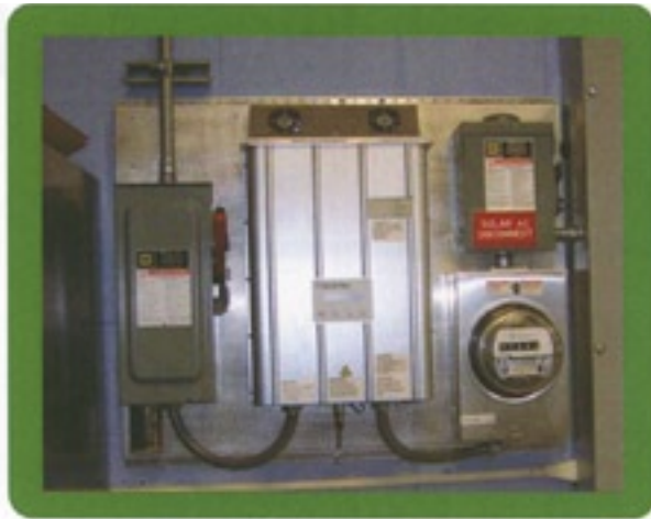
The solar inverter in the Murchpy school science lab
